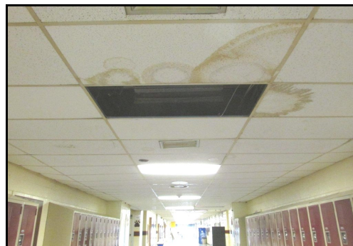
Gaping Leak in the GHS Hallway
