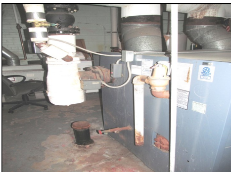
40-Year-Old Boiler at J. Harvey Rodgers School
