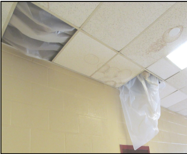
Large Ceiling Leaks at Thomas E. Bowe School
